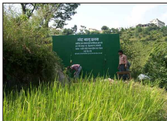
Slow Sand Filters designed, constructed and commissioned by NEERI at village Chhati in hilly region of Tehri Garhwal
