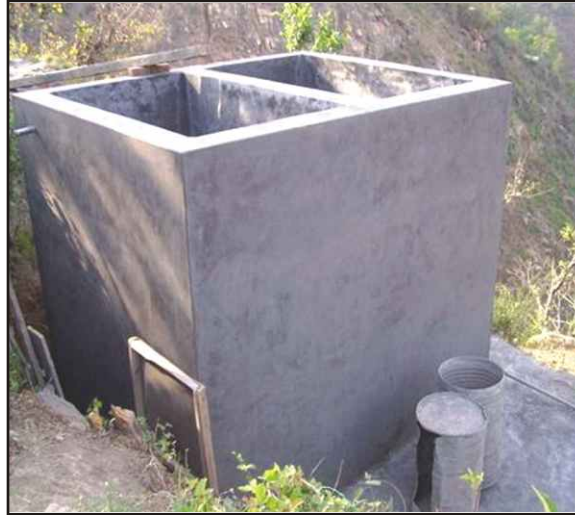
Slow Sand Filtration Unit under construction at village Chhati, Tehri Garhwal, HP
