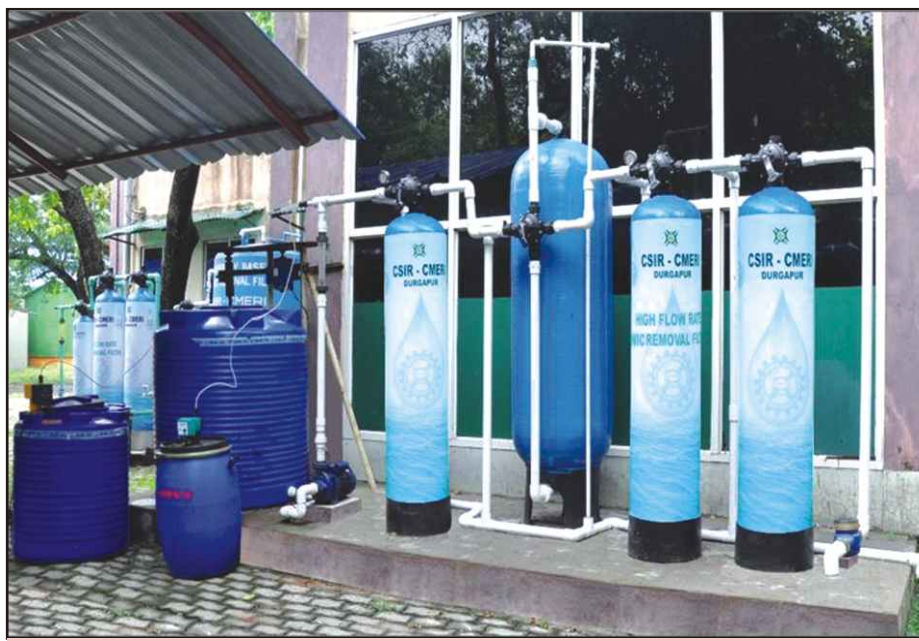
High Flow Rate Arsenic Removal Filter at CSIR-CMERI
