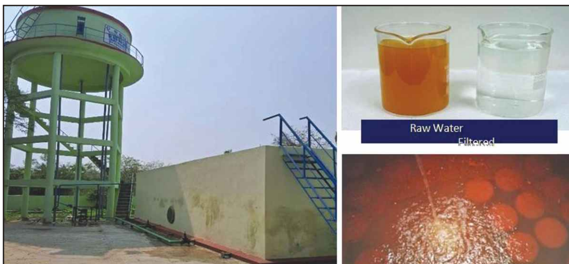
Fig 8. (a) 60KL/day TERAFIL Filter plant; (b) Source water inside TERAFIL Plant with filter media; (c) Raw water and product water quality.
