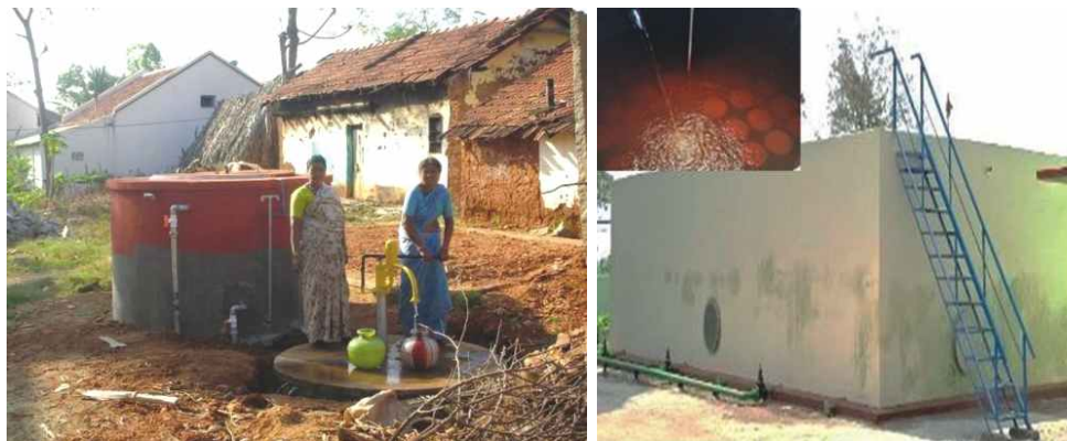
Fig 4. RCC based TERAFIL Filtration unit
