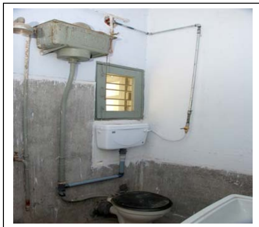
Grey water for toilet flushing
